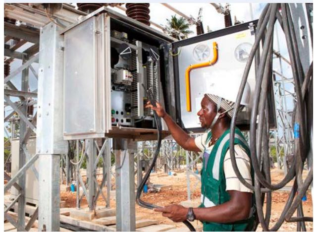
MCC Tanzania expanded electrical infrastructure by connecting the Zanzibar Archipelago to the mainland via an undersea cable. Credit: MCC
