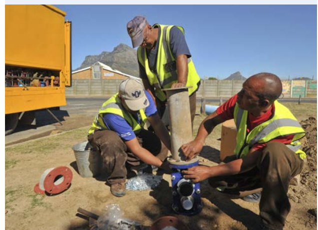
USAID South Africa's water supply work in Cape Town aims to diversify the city's water supply and reduce risks from drought. Credit: USAID
