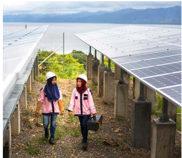
Electrical technicians inspect and maintain solar panels on Karampuang Island, Indonesia, to extend the life cycle of the energy infrastructure. Credit: MCC
