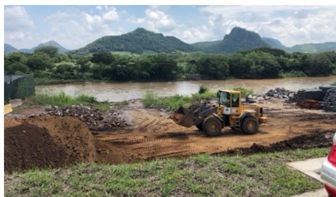
Land clearance work at El Amatillo in preparation for construction of new freight border facility.
