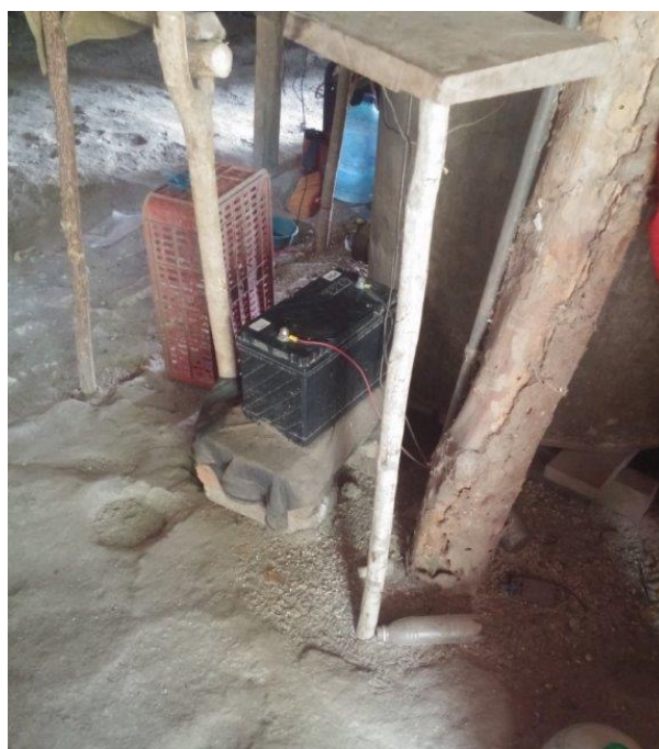
Battery of a solar panel installation
