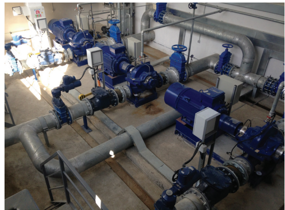
Rehabilitated pumping station in Lopatna Centralized Irrigation System
