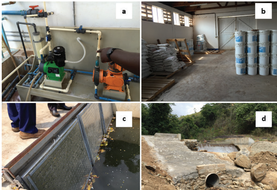
(A) REPAIRED PRE-DOSING PUMP AT MAFIGA; (B) CHEMICAL SUPPLIES AT MAFIGA; (C) NEW STRAINERS INSTALLED AT MAMBOGO IN-TAKE; (D) LARGER WASHOUT PIPE INSTALLED AT MAMBOGO
